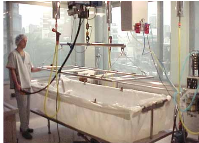
FIGURE 6. Burn Unit Hydrotherapy Room and Mechanical Transportation System by Crane
