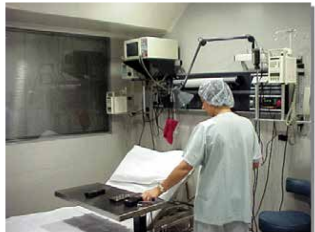
FIGURE 4. Burn Unit Patients Rooms, Fully Equipped
